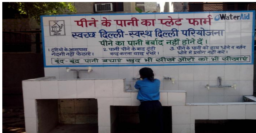
Three stage drinking water point at school
